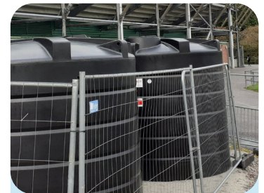
Above ground water storage tanks at Plymouth Argyle
